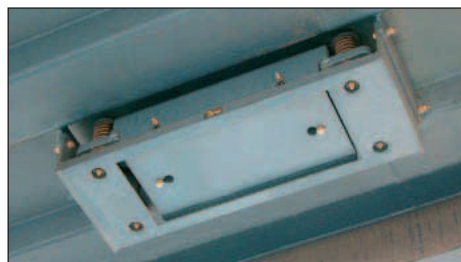
Abb. 1: Passiver GERB Schwingungstilger (GERB Brückentilger – Britzer Damm, Berlin)
